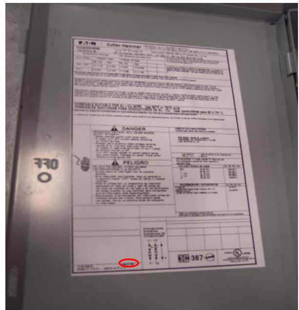
Figure 3: The red circle indicates where the date code is located on the pub inside the case of the switch
