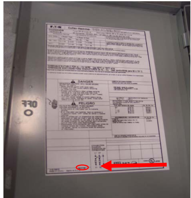
Figure 3: The red circle indicates where the date code is located on the pub inside the case of the switch
